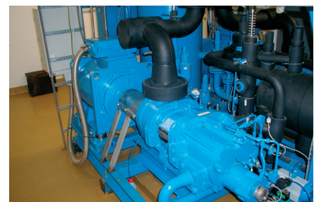
Ethyleneglycol chiller unit
